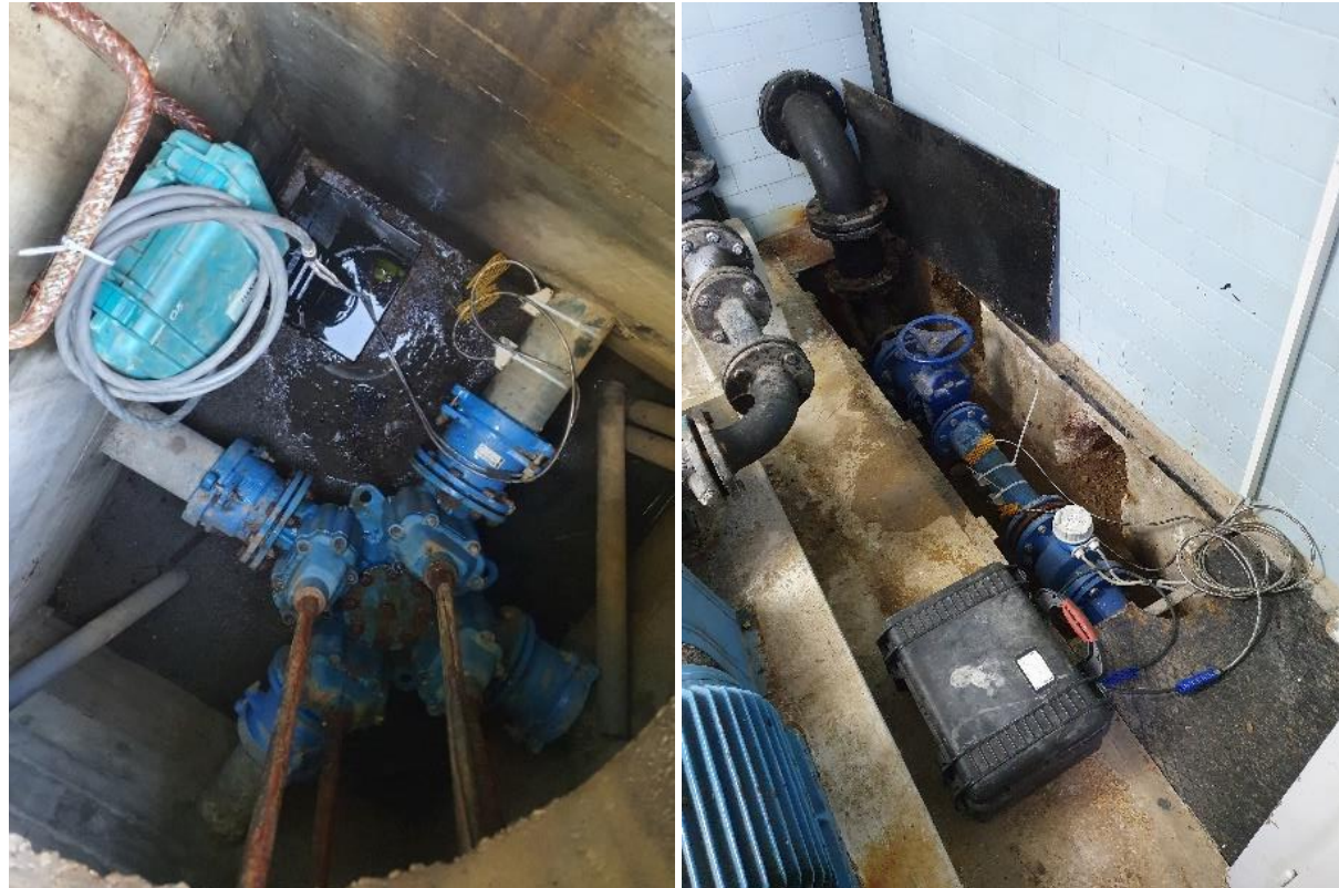
Flow measurement using ultrasonic flow meter
